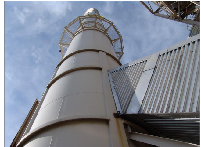
Source: Emerson Industrial Automation
